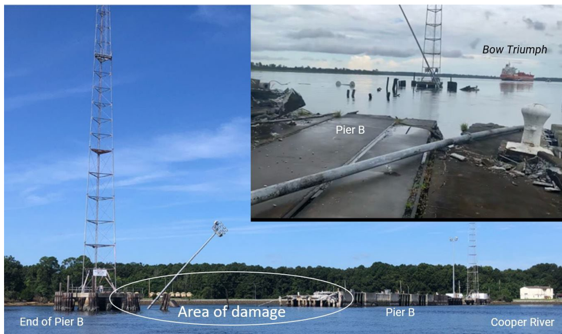
Figure 7. Pier B damage. Inset: Witness photograph taken shortly after the contact. (Sources: Corps of Engineers, Jacob Wall [inset])
